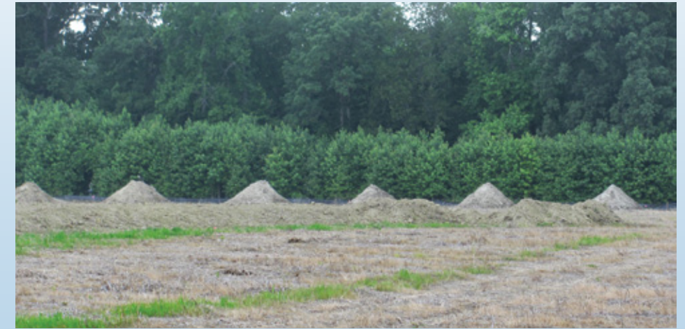
Topsoil is piled before the wetland is dug out and then placed on the berms to encourage plant growth.
